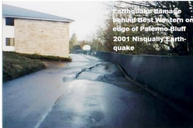
Figure 1: The Best Western hotel located on the bluff above the Palermo well field had a portion of the rear parking lot settle and start to slide down the hill. (Former Tumwater Fire Chief John Carpenter-phone conversation 6-3/9/10-2009)
